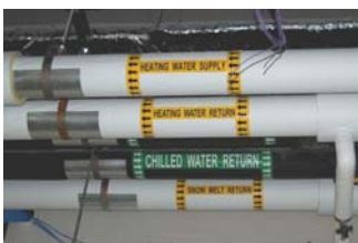
Pipes are installed and labeled above the ceiling tiles.
