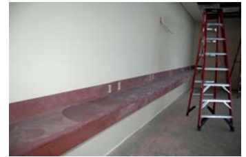
Installation of the countertop in the Business Center is complete. The Center will have seating and ample power outlets for charging devices.
