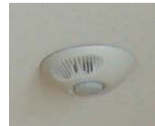
Sensor in an office ceiling.
